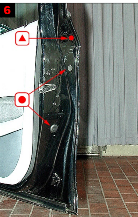
6 Front door: Door - top member. Treat via 1 drilled hole. Remainder via existing plugged holes.
