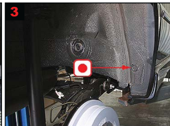
3 Wheel arch rear/panel: Treat via existing plugged hole.
