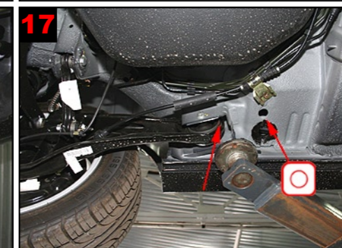
17 Longitudinal member before wheel arch rear and reinforcement: Treat via existing holes and gaps.
