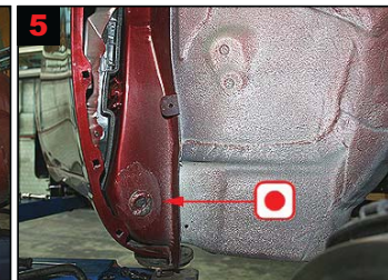
5 Wheel arch front/panel: Treat via existing plugged hole.
