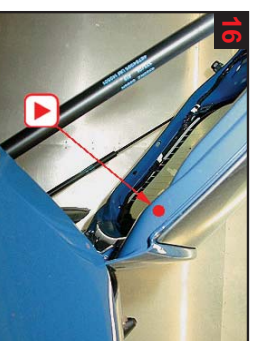
Tailgate side by roof: Treat via 1 drilled hole.
