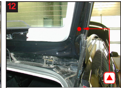
Tailgate side by roof. Treat via 1 drilled hole.
