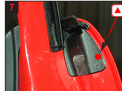
Door - topmember. Treat via 1 drill hole just above clips for cover plate.
