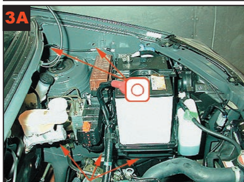
3A Engine compartment sectional view, left side: Treatment of top members in wings, on top of longitudinal members, under fluid reservoir, ABS distributor.
